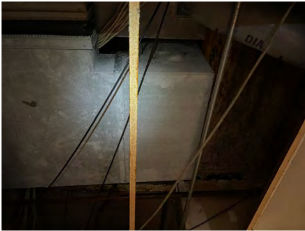
3 rd Floor Above Ceilings
